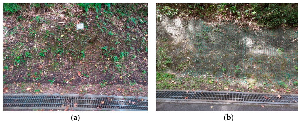
Figure 6. Application of the sugar palm fiber net (a) and a common synthetic net on (b) the embankment near the front of the main entrance of the RIHN building.
