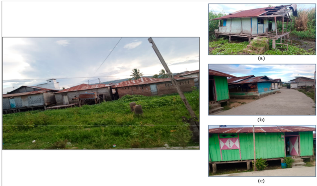
Figure 7. Impoverished conditions of one village at the rear of the permanent house is built of brick. (a) Deteriorated plank house, (b) permanent houses, and (c) low-plank house.
