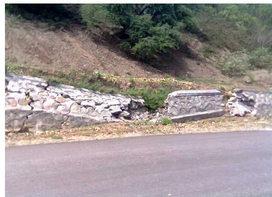
Gambar 7. Keruntuhan dinding penahan tanah (Foto dok. Achmad).
