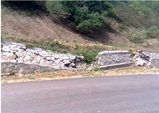
Gambar 4. Keruntuhan dinding penahan tanah (Foto dok. Achmad).
