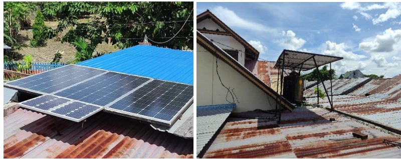
Fig 10. PV installed on the carport's roof (left), and on a rack (right)
